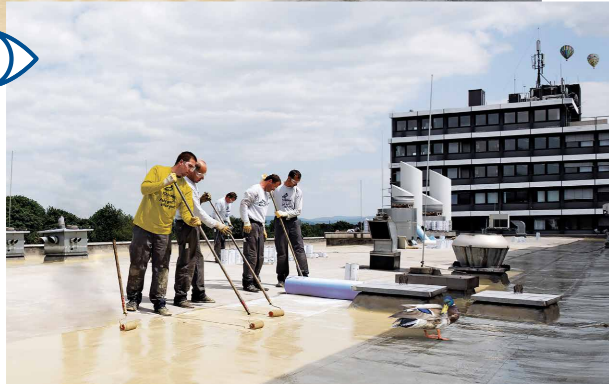
Application of KEMPEROL on the roof of the HNA printing centre Kassel, 2008.
