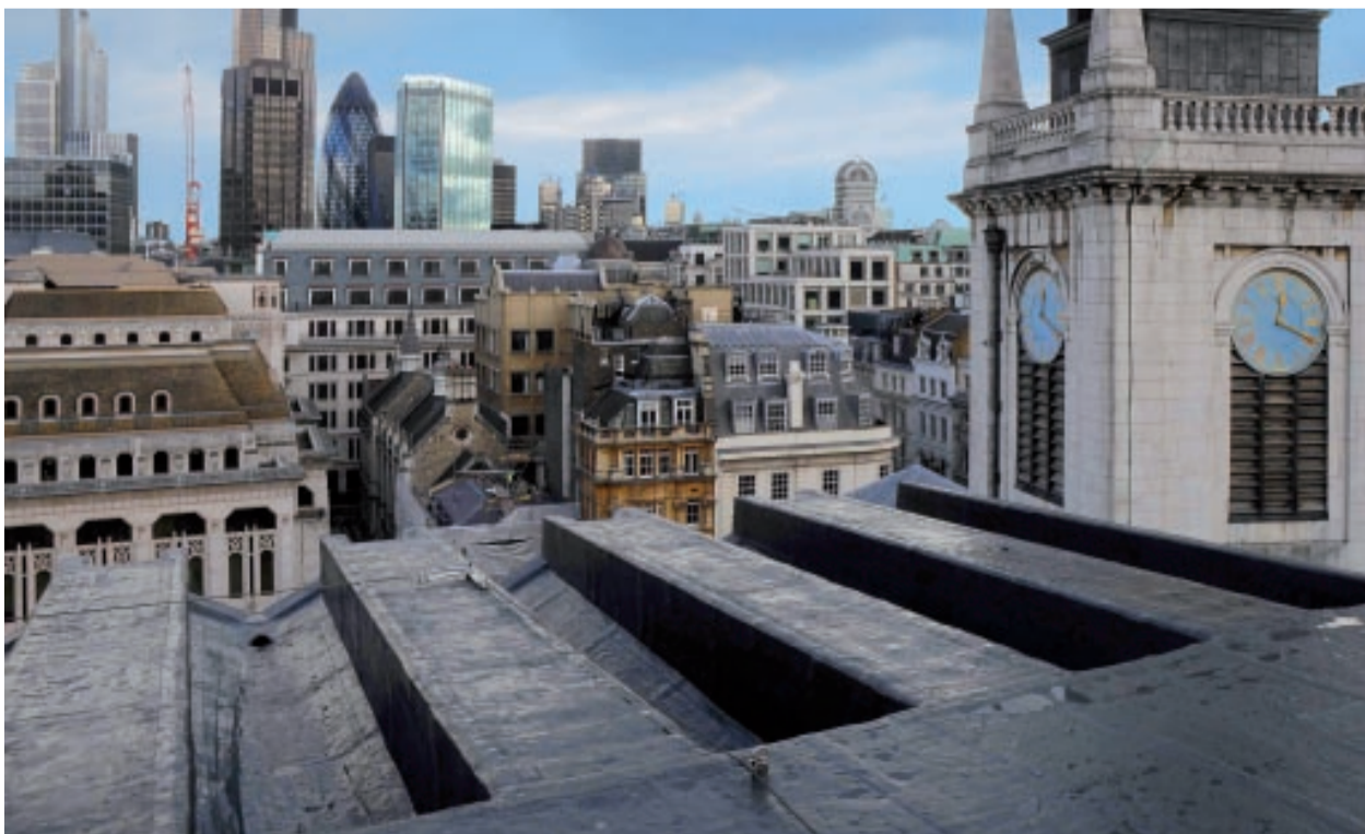
Deep drainage channels extending out from the central spine of the roof
