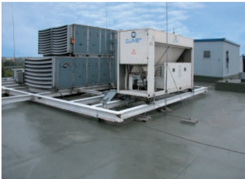
A special challenge was the application of liquid waterproofing underneath the air conditioning system. The installation height was just 15 cm.
