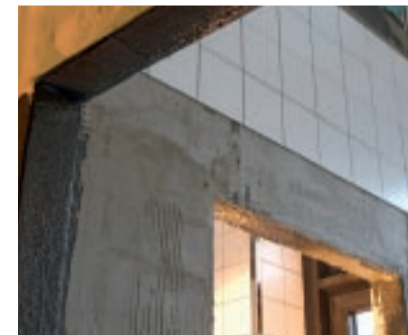
All the phases can be seen in this photo: the waterproofing in the corridor, the levelling layer and the tiles on the wall.
