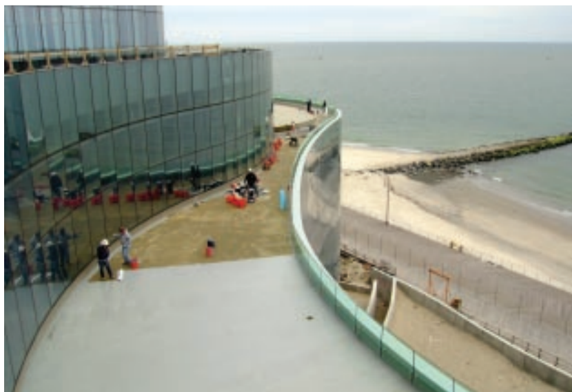
Sealing the View: The top layer of CFA resin is rolled out over the fleece membrane on a sweeping walkway to be topped with pedestal pavers. Along the outside curbs, special tempered glass maintains the view, and on each sheet of (inside) guard rail, the four anchor bolts were field flashed with the KEMPER SYSTEM.
