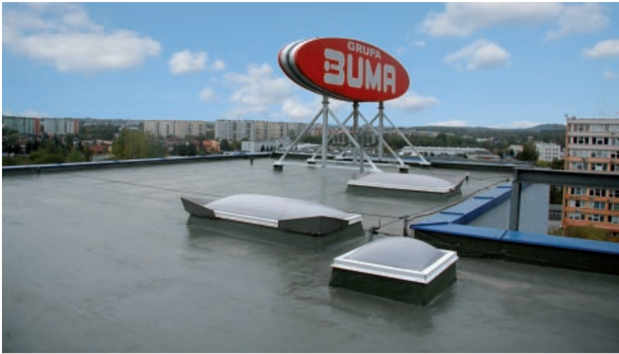
The roof of the Buma Square Business Park in Krakow was waterproofed using odourless KEMPEROL® 2K-PUR.
