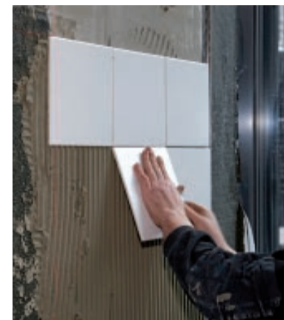
The tilers applied a levelling layer before gluing the tiles in place.
