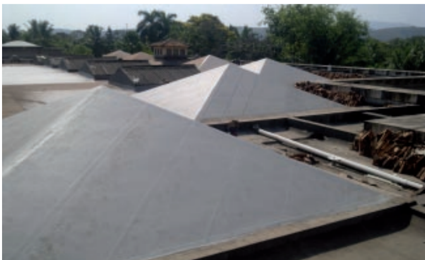
The waterproofing is applied directly onto the failed material easily and quickly.
