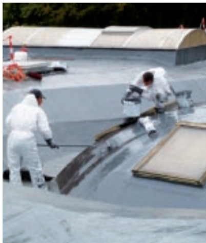
Fabricated on site: The liquid resin adapts to every substrate and structural detail.
